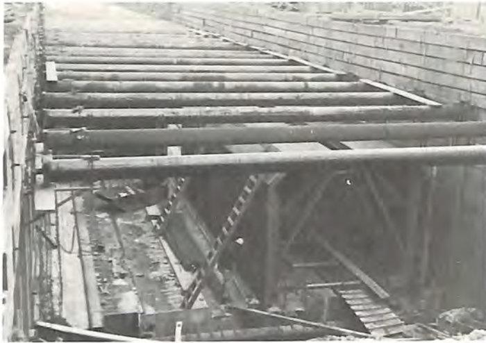
Subway construction in Oakland; steel form for subway shell in place on right.
