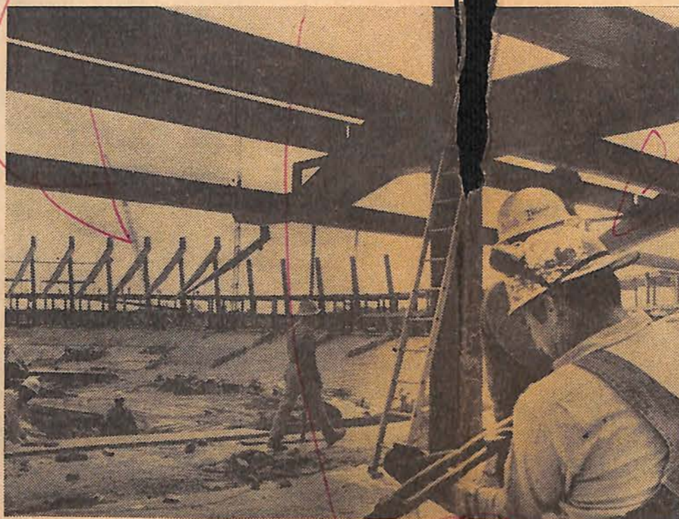
NEW HOME FOR BRAVES? Workers at new stadium in Atlanta. The Milwaukee Braves will ask the National League owners for permission to move their franchise there.
