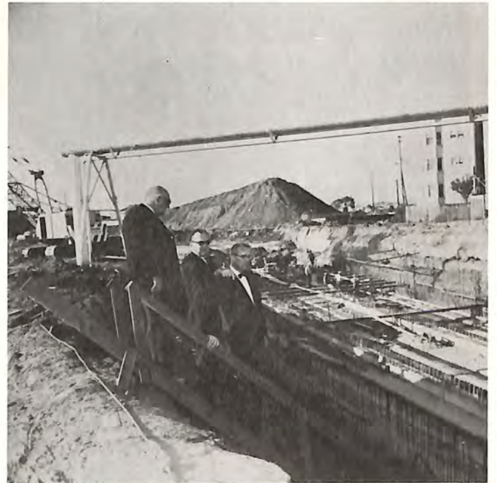
Robert L. Sommerville (L), John Coil, and Henry Stuart look over subway construction work in San Francisco. Overhead is a gas pipeline which has been re-routed during subway construction.
