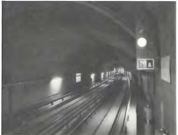
Tunnels on the Metro are lighted all the way for safety and comfort. Note the signal (upper right) that provides the train operator with indications about the track ahead.
