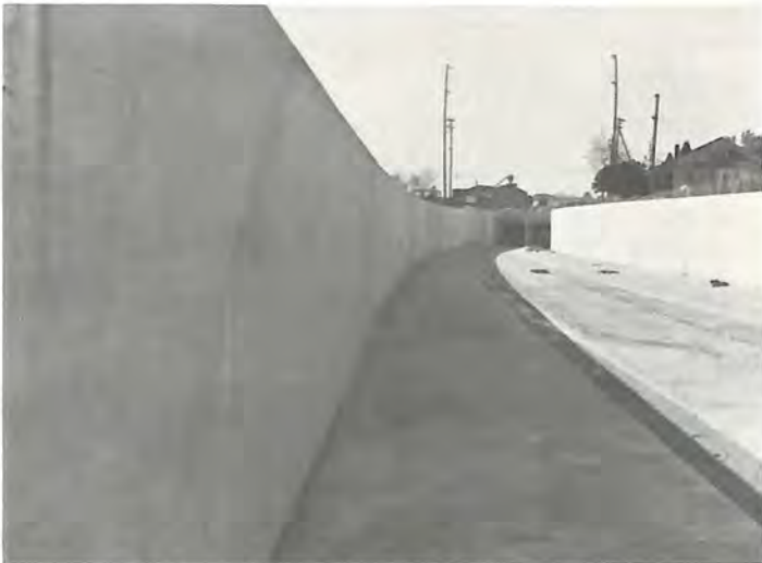
Almost-completed construction on transition section of subway; construction goes from cut-and-cover subway to ground level track.
